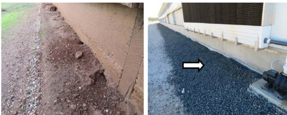
Image 6: Norway rat burrows along the edges of a structure (left); road base gravel laid down to prevent burrowing (right) (Brown and Henry, 2018).
