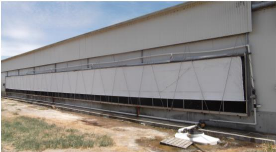
Photograph 7 - Cooling pads from outside of layer shed
