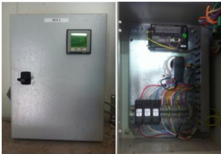
Photograph 11 - Nemo 72-L Power Meter and Logger
