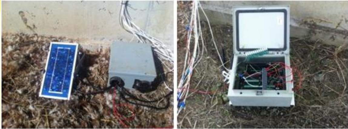
Photograph 13 - Fan activity data logging equipment
