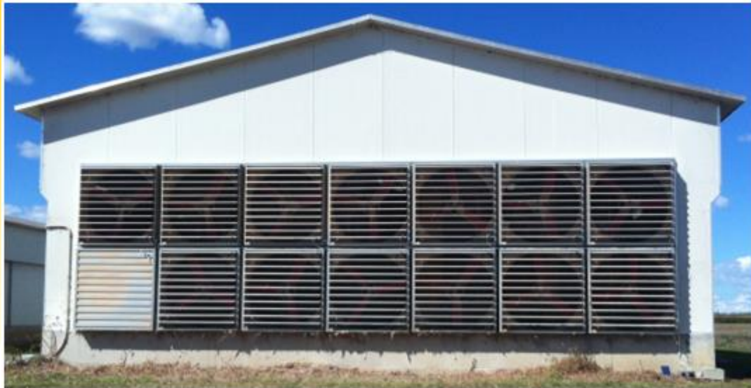
Photograph 5 - Tunnel ventilated shed - exhaust fans
