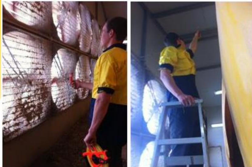
Photograph 22 - Fan cross sectional performance data collection
