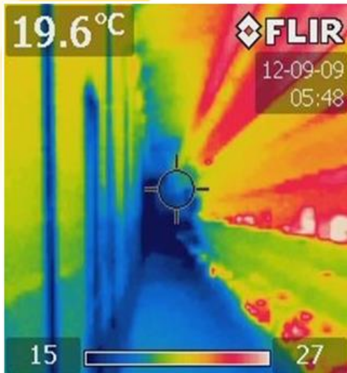
Figure 4-31 - Inadequate mixing of cold air with warm air during September trial
