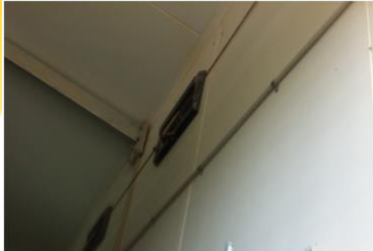
Photograph 6 - Inlet vents alongside of layer shed
