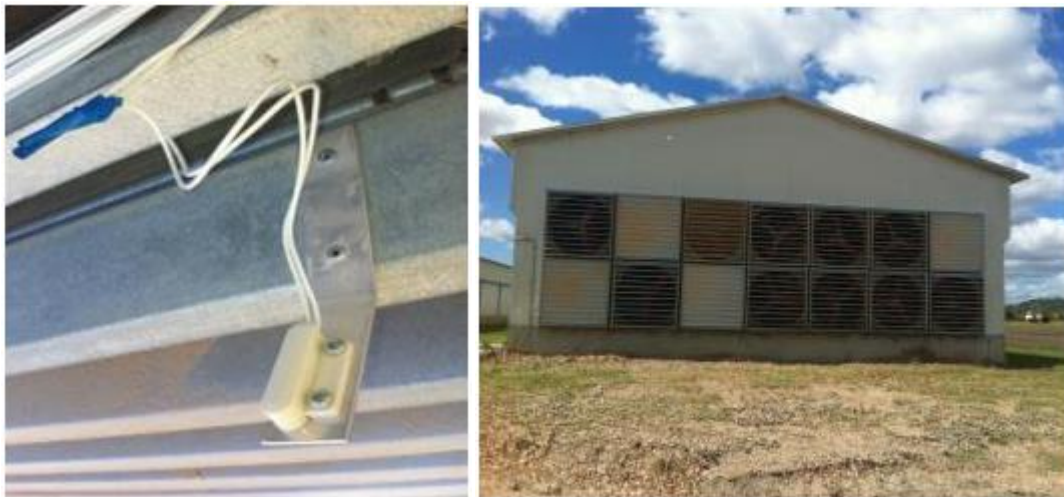
Photograph 12 - Mercury tilt switch (left) and shed exhaust fans (right)
