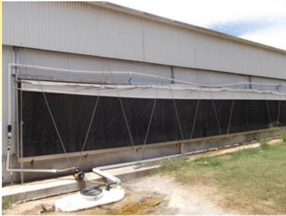
Photograph 8 - Shed 5 cooling pads
